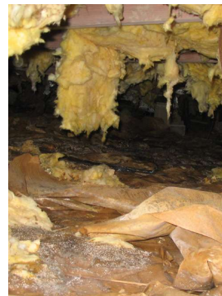
Insulation in the crawl space is falling and in need of repair.
