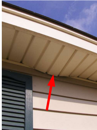
Loose siding on the east side of the home.
