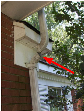
Damaged downspout observed on the northwest corner of the home.
