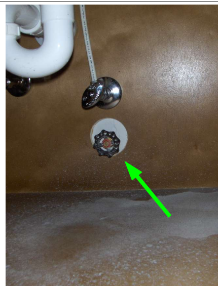
Main water valve located in the first floor hall bathroom.
