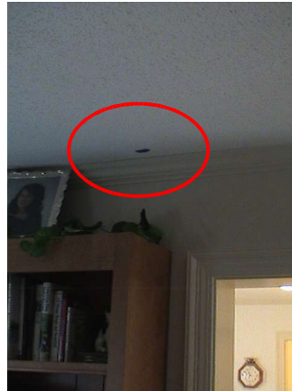
Waste line leak on the living room ceiling.
