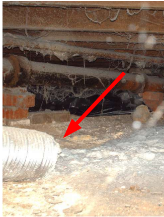
Dryer exhaust vent terminating in the crawl space.
