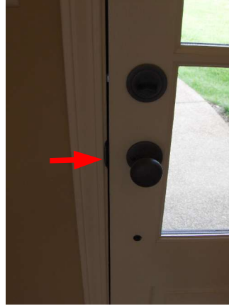
Mis aligned door latch and striker plate on the front door.
