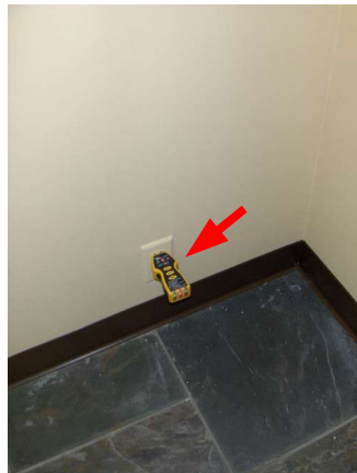
Hot and neutral wire reversed on outlet in the laundry room.
