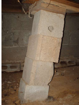
Damaged column in need of repair.
