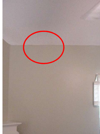
Roof leak in the area of the living room.
